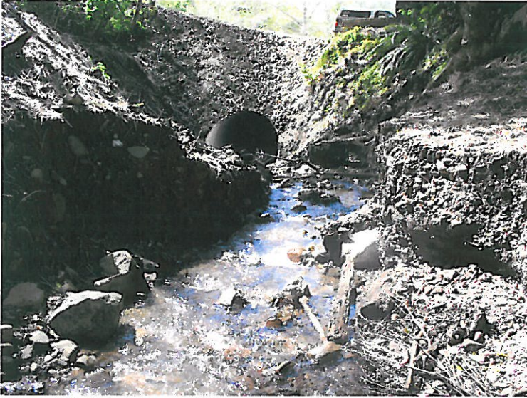
Figure 11: Inlet of one of the county culverts (on both forks) upstream of U.S. 101.
